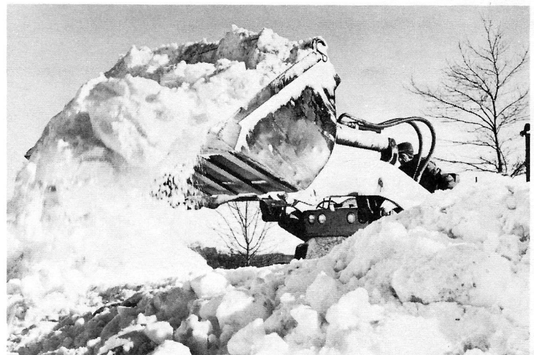
Route 22 near Indiantown Gap, Lebanon County cleared for two-lane traffic. Snow had to be removed rather than plowed in many areas.
